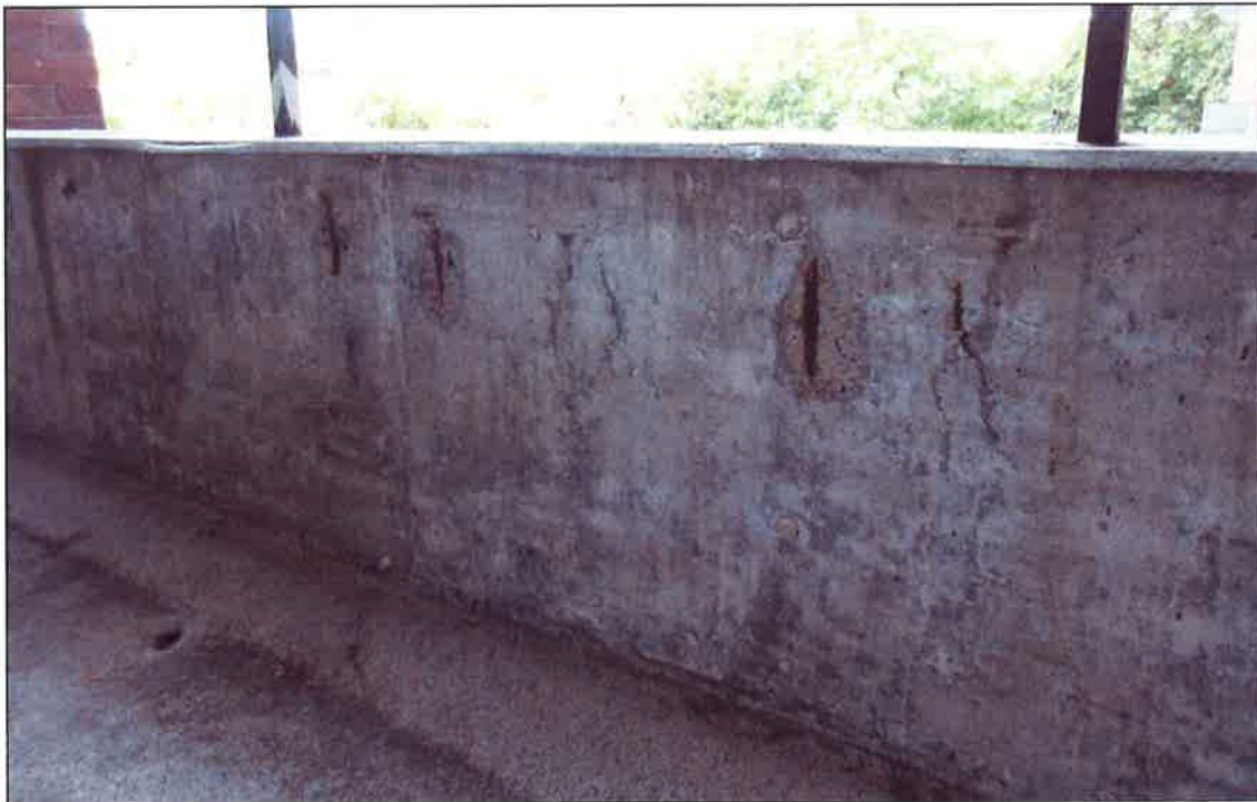
Photo 6 – Spalling Concrete and Corroding Rebar
