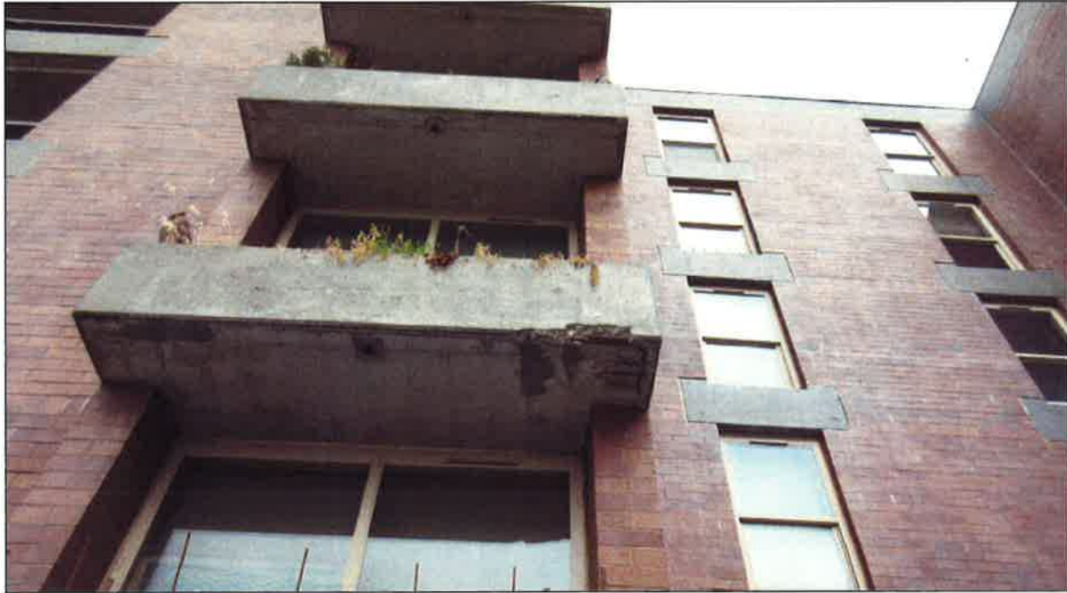
Photo 2 – Spalling Concrete with Exposed Rebar and Previous Patches on Planter
