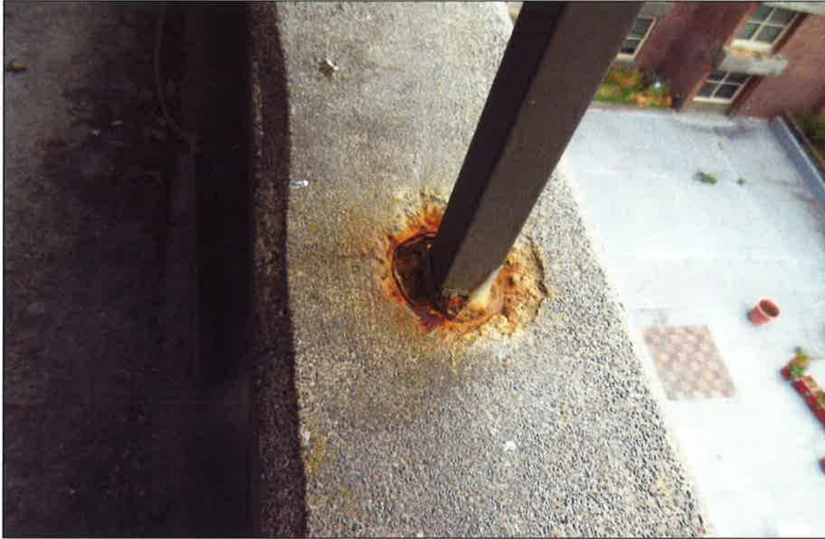
Photo 7 – Corroding Deck Rail
