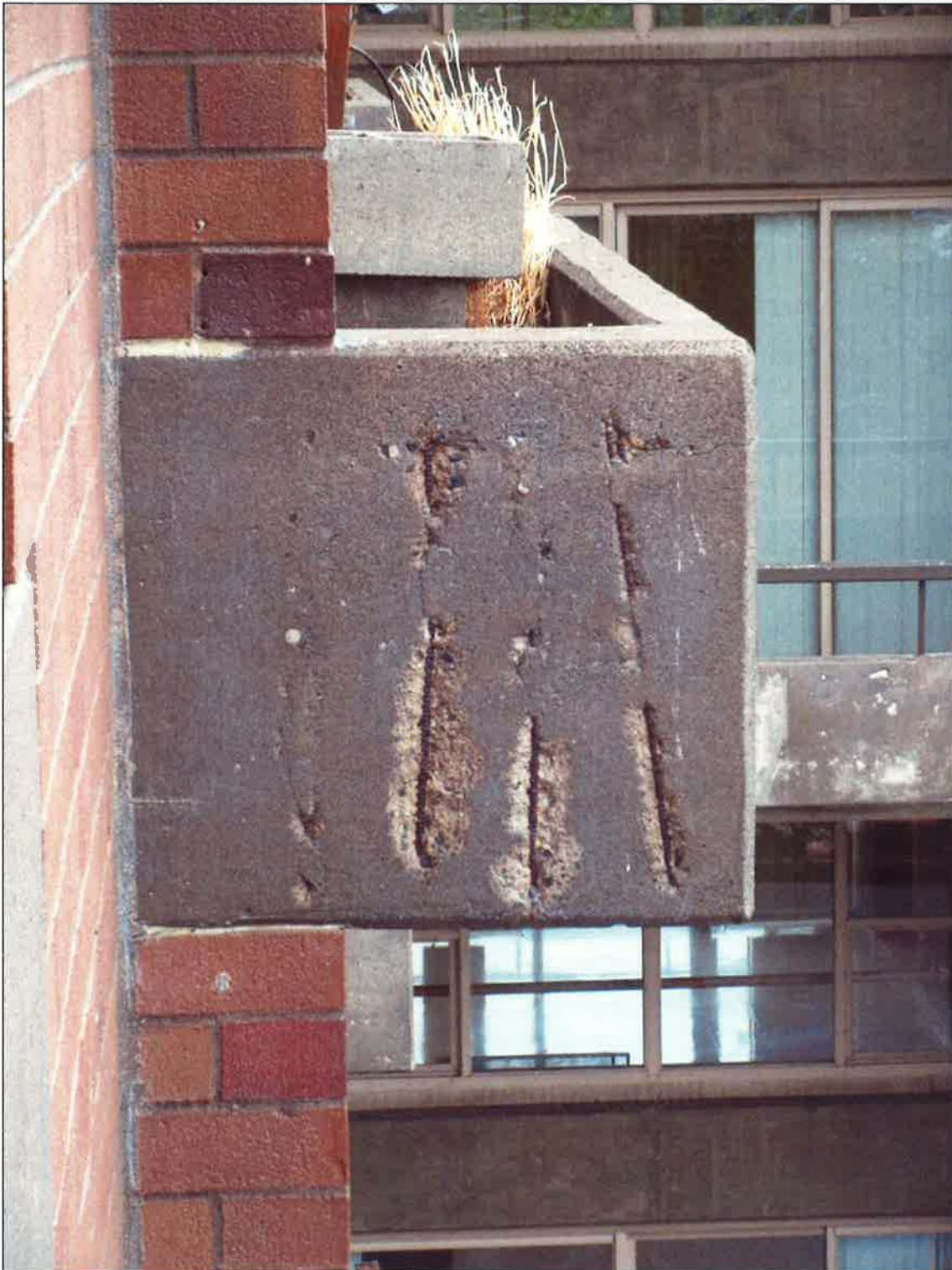
Photo 4 – Spalling on Side of Concrete Planter
