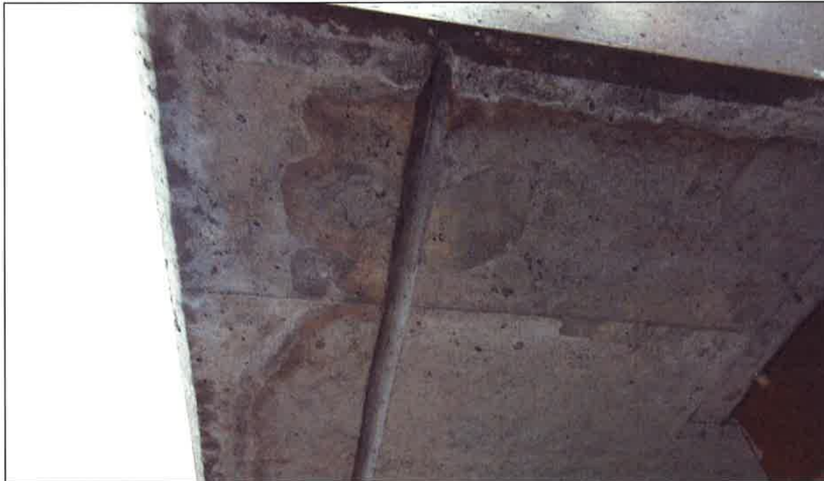
Photo 3 – Water Staining on Planter
