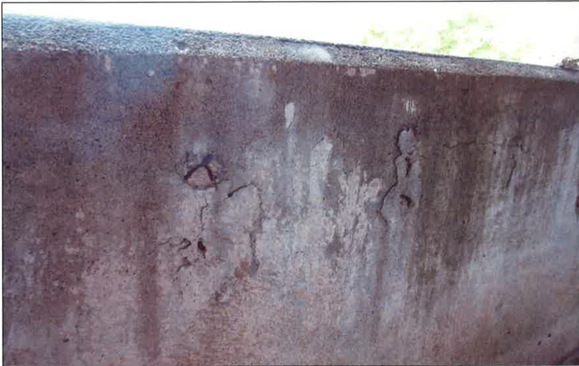
Photo 5 – Rusting Wire Ties and Spalling Concrete
