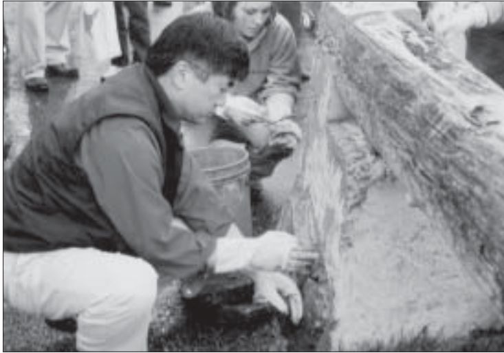
Gov. Gary Locke and an AmeriCorps member apply mortar to a wall at Saltwater State Park.
